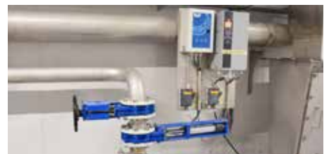
AVK knife gate valves with linear actuators on a reject water pipeline. The linear actuators were chosen, since they are energy efficient compared to actuators using compressed air
