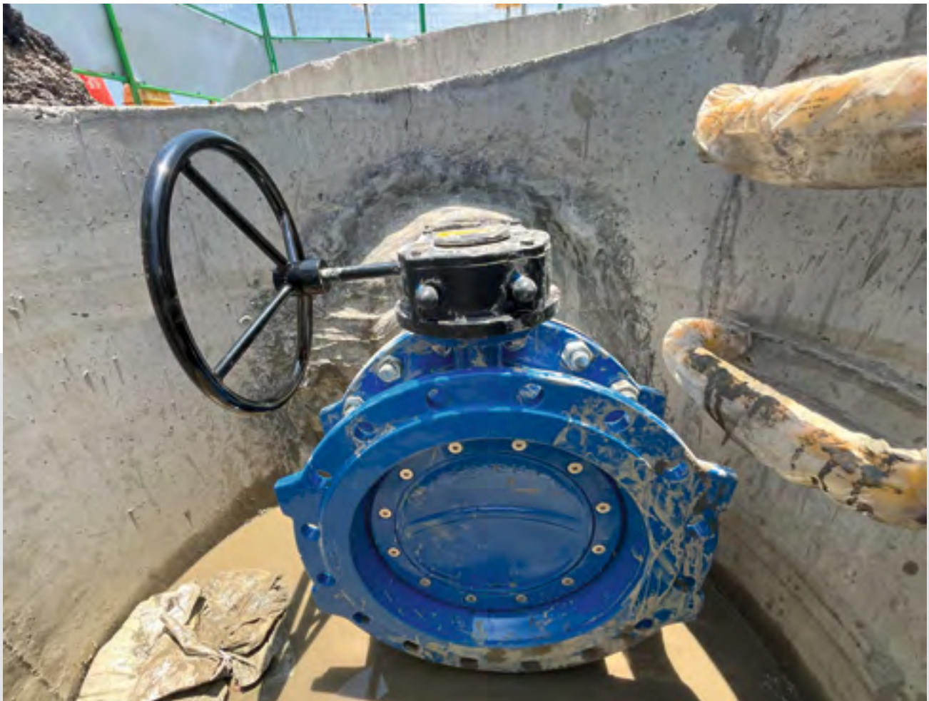
Butterfly valve installed
