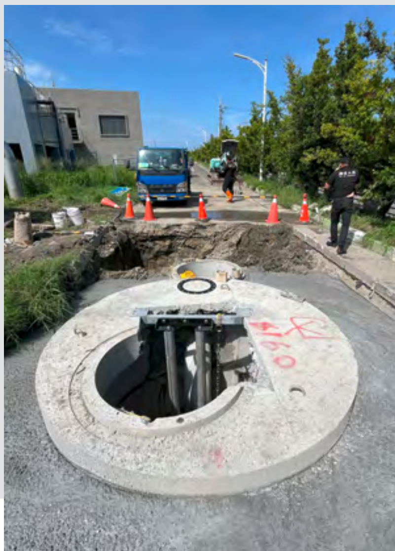
Valve installation location
